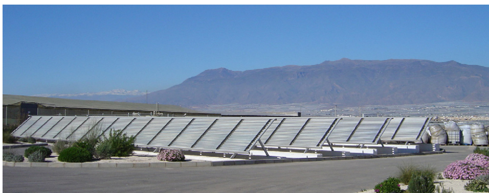
Fig. 8. View of the solar detoxification demonstration plant erected by ALBAIDA at La Mojonera (Almería, Spain).
